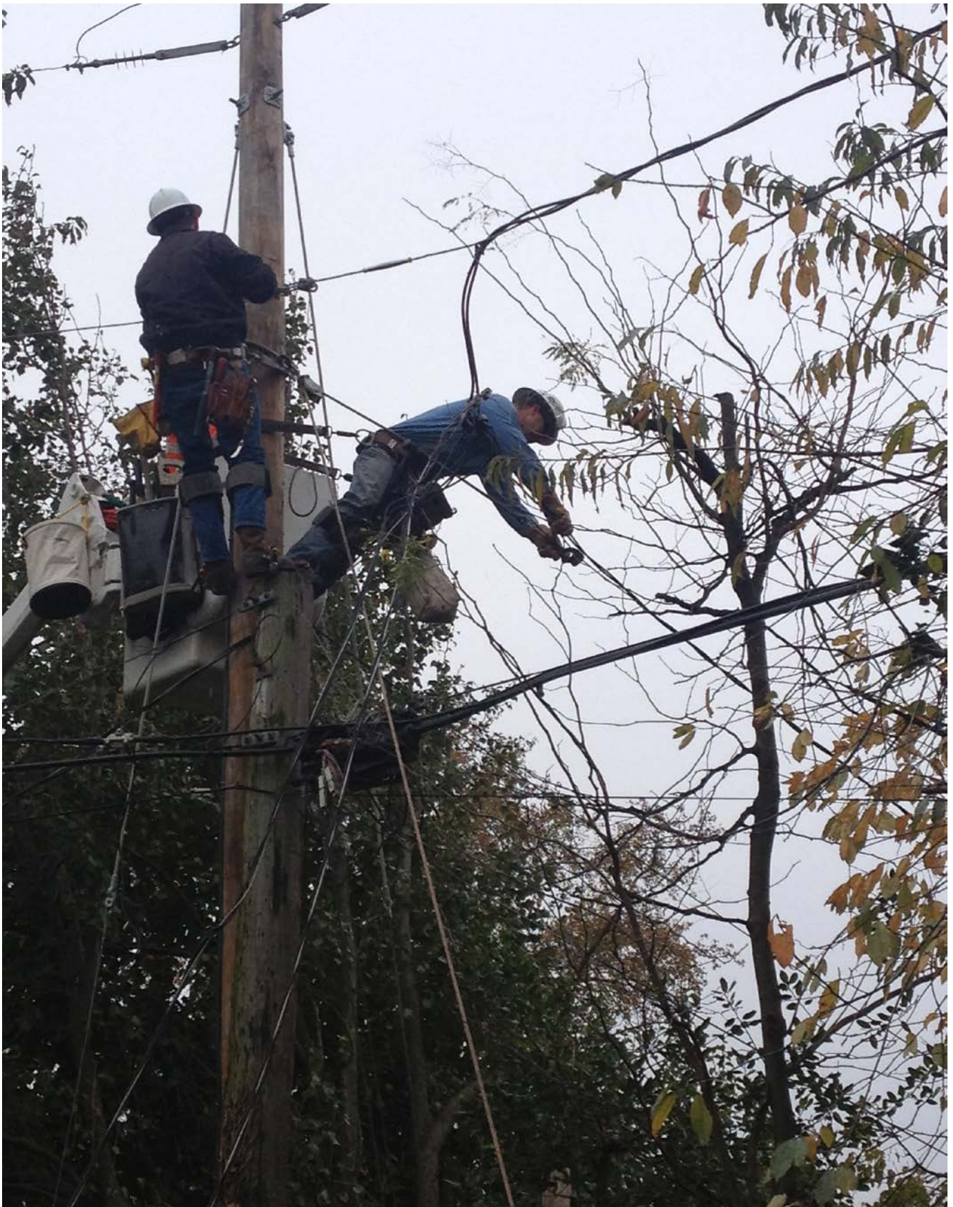
Photo courtesy of Kissimmee Utility Authority, Florida
